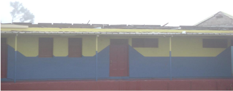
Manning's Boys Home in December 2007 after Hurricane Dean
